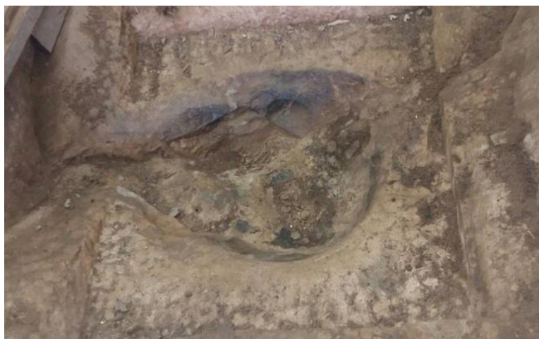
Fig. 9 - The stone laqân in the Abu Seifein church at Dayr of El-Maimum, in a bad situation. (©Author's photography)
