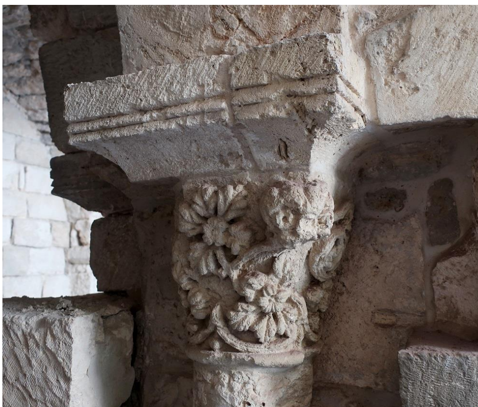
Fig. 5 – Cloister of S. Maria Latina (today Church of the Redeemer), capital, ground floor of the east wing (photo: Dorothee Heinzelmänn, 2019).
